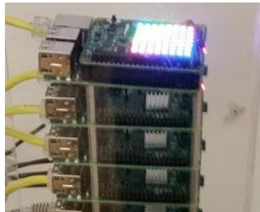
Figure 5.2: Sense HAT installed on MADNS.
